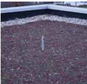
ParaSave P1 Fall Protection – installed
